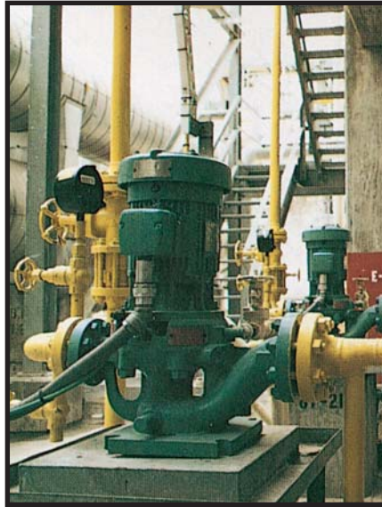
LMV-802 Pumps in Gulf Coast Refinery.
