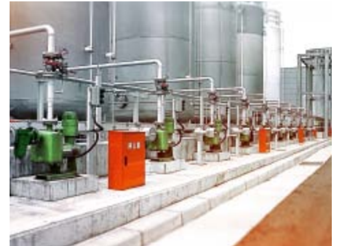
Self-priming type pumps in a paint manufacturing plant.
