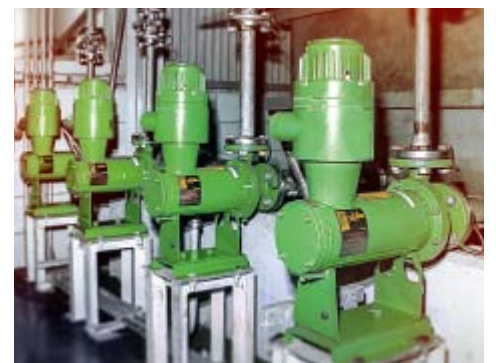
Basic type pumps in a chemical plant.
